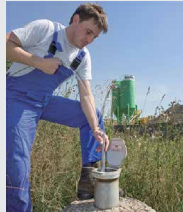
Installation of Data Logger
